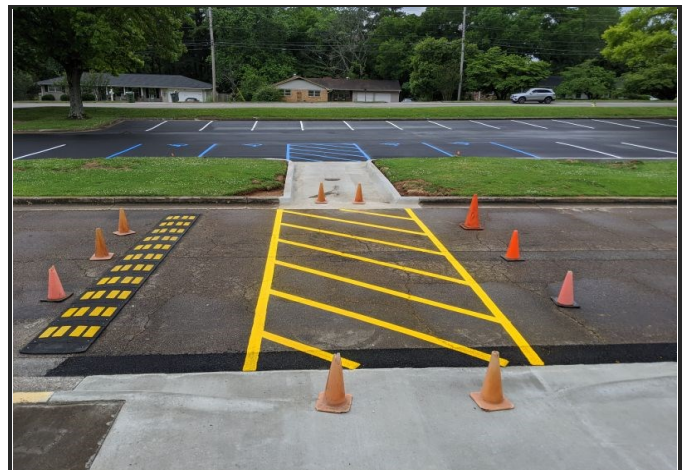
Striping is complete. Next we will be adding new parking and directional signs.
