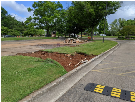
Making sidewalk accessible by lowering to parking lot/drive level. Curb to be cut and removed as well.
